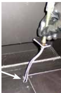
Light assembly wiring
