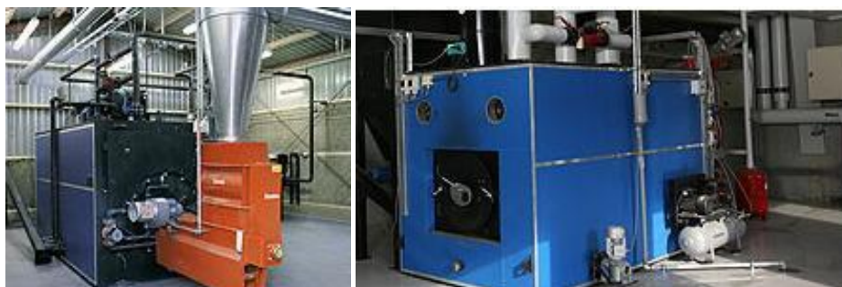
Figure 7-10: Biomass Briquette Systems LINKA Energy 25
