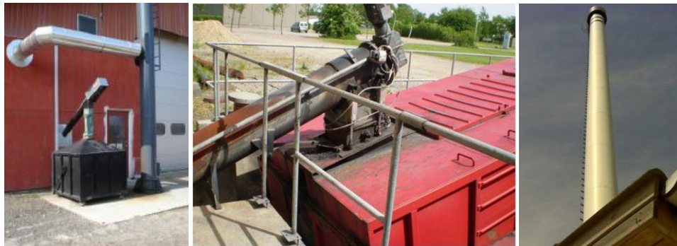
Figure 8-6: Ash and Soot Handling
