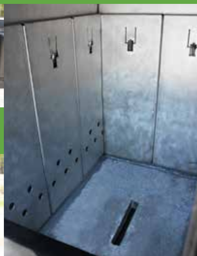
Air Panels & Gasification Manifold
