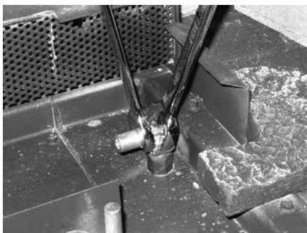
Burner Orifice Removal
