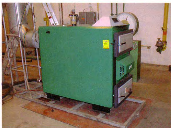
Fig. 2 - overall view of the boiler
