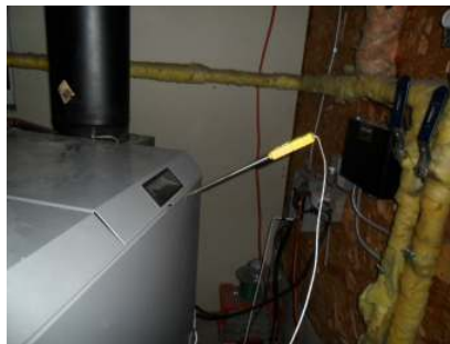
“K” type thermocouple measuring chimney smoke temperatures
