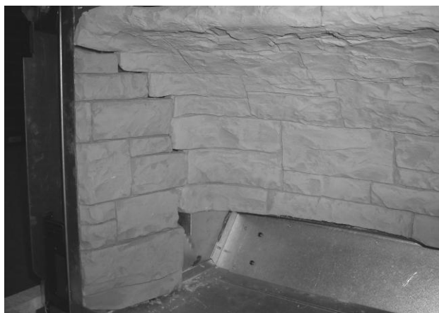
Photo 2 - Left Baffle Panel
