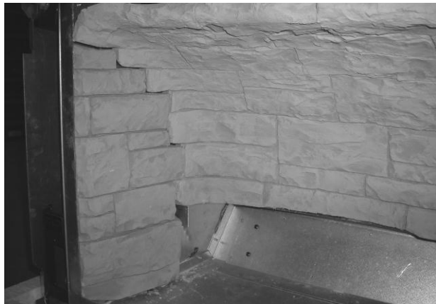
Photo 2 - Left Baffle Panel
