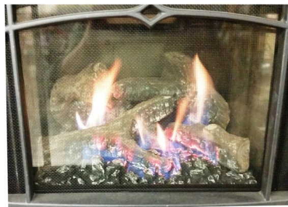
Figure 40 – Typical Burner Flame Appearance
