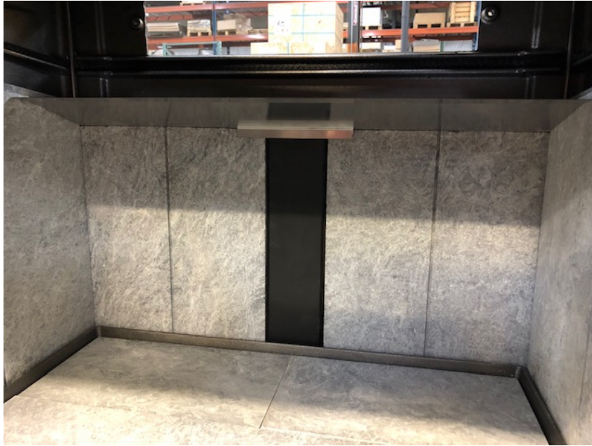
Photo 5. Secondary air riser installed.
