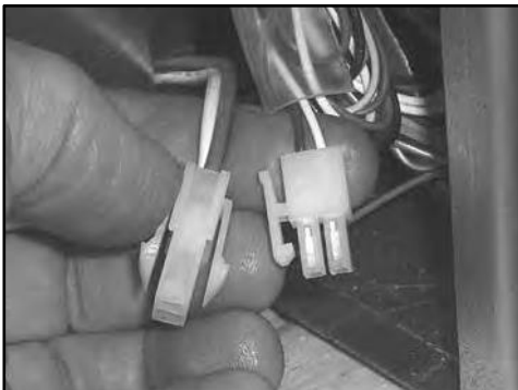
Figure 14: Disconnecting Standing Pilot Switch.
