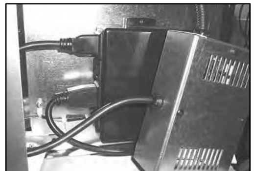
Figure 17: Plugging PVK into Electric Box.
