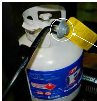
Gas connection @ tank
