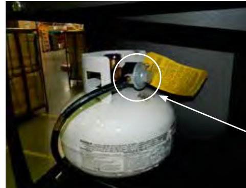
Gas connection @ tank
