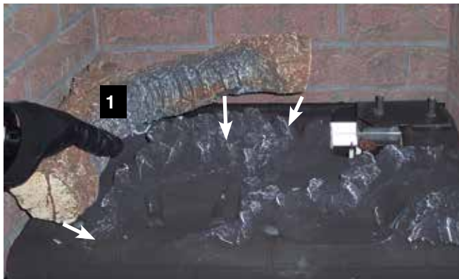
Log 1 location on burner
