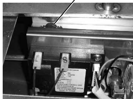
Limit Switch Location
