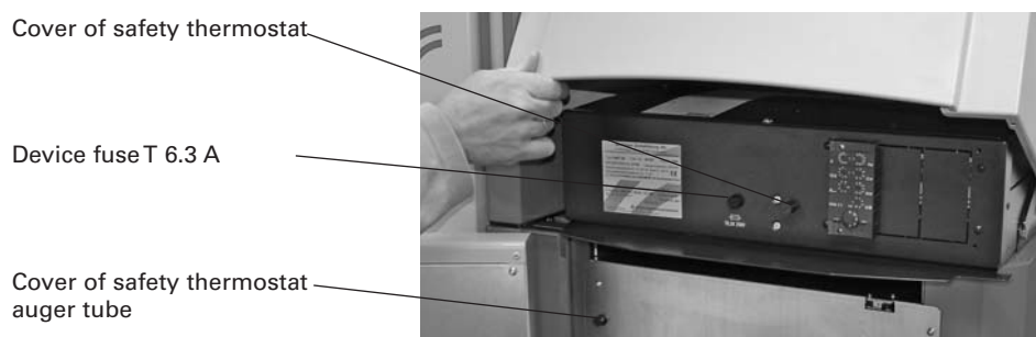
Fig. 146 BioWIN control panel cladding raised, combustion chamber door open
